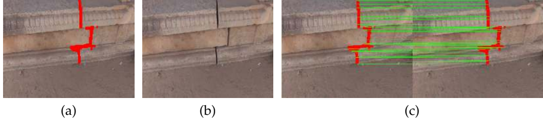
Figure 7.20: Tracking detected regions using the estimated homography matrix. (a) Detected damaged regions in the frame f_{i-1} ; (b) frame f_i ; (c) tracked cracks in the frame f_i . Green lines show the mapping of few points on the boundary of crack regions, while the detected and tracked cracked regions using SIFT features are shown in red.
