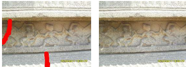
(a) Input image I overlaid with the crack detected in I_g shown in red color (b) Inpainted version of I using the region detected in I_g in red color
